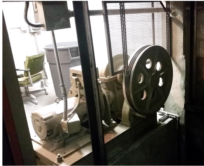
Elevator pulley and cable.
